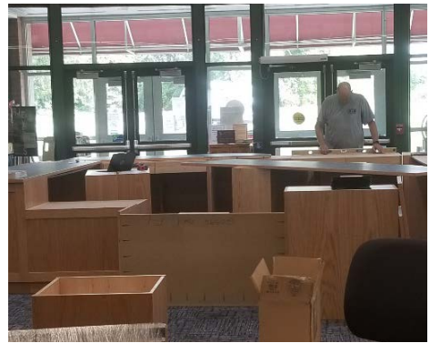
Installation of the ADA accessible circulation desk, thanks to a generous donation from the Friends of the RJCL
