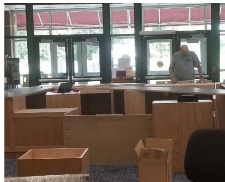
Installation of the ADA accessible circulation desk, thanks to a generous donation from the Friends of the RJCL
